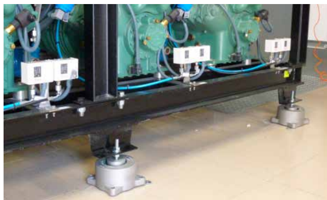
Example of installation on a HVAC equipment
