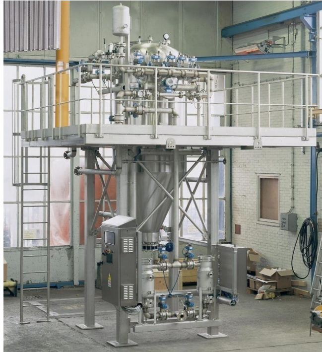
Fully automated Cricket Filter station with included polish filters
