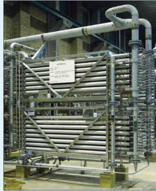
View of feed end of sixth stage of hardwood line. Note: Larger diameter feed pipework
