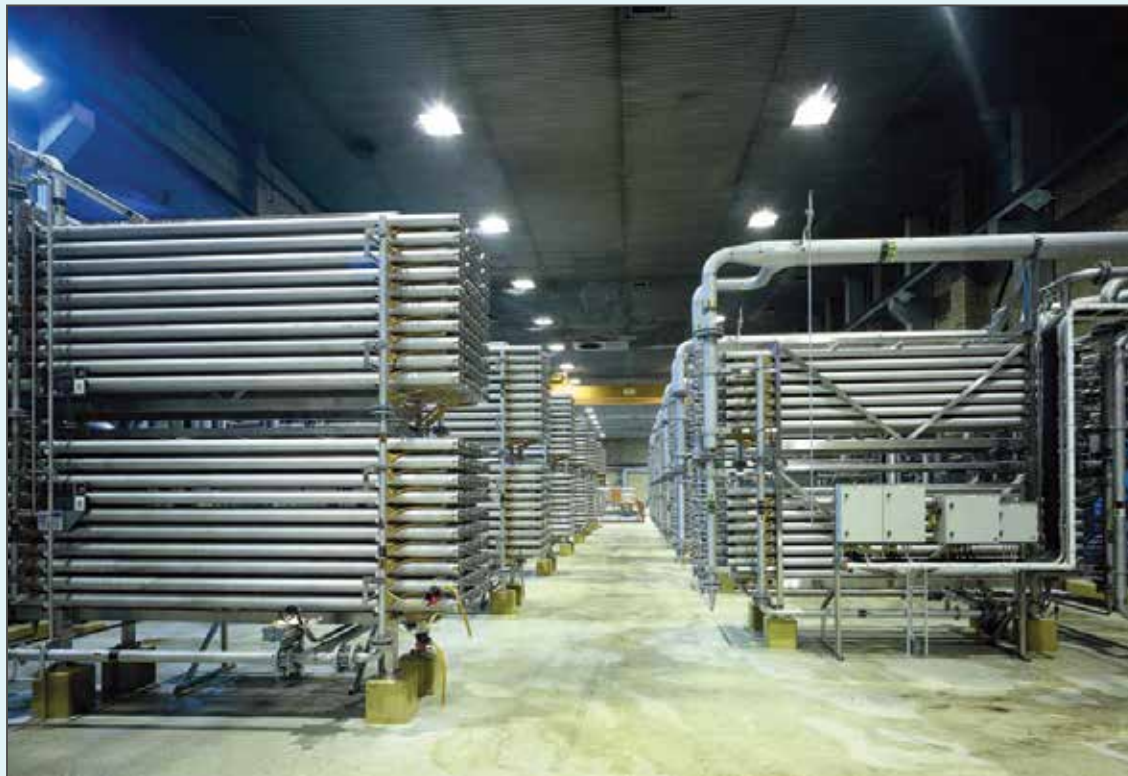
13 stages of PCI 3.6 m long B1 modules. A total membrane area of 4650m 2 . Note: Stages are staggered to make space for re-membraning.
