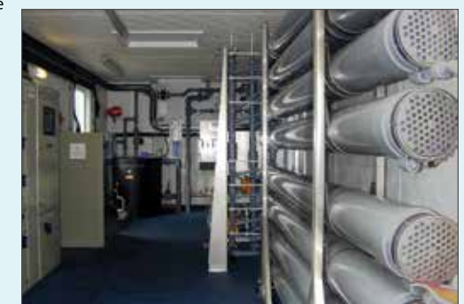
Interior photo of the package membrane plant
