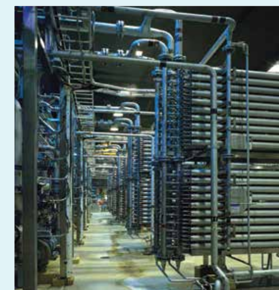
View of feed end of softwood stages. Note: Small diameter pipework – a feature of operating at low cross-flow rates.
