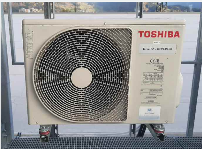
External air-handling unit on wall bracket
