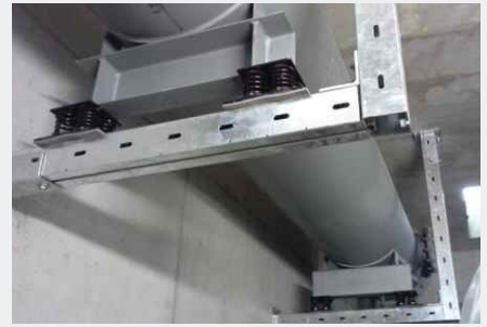
Bearing of duct silencer
