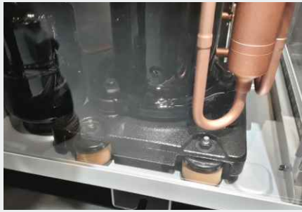
Bearing of a compressor assembly on an internal frame
