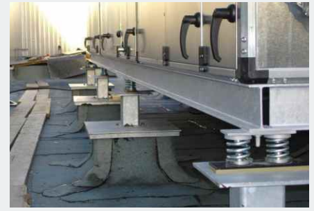
Roof-mounted AC system
