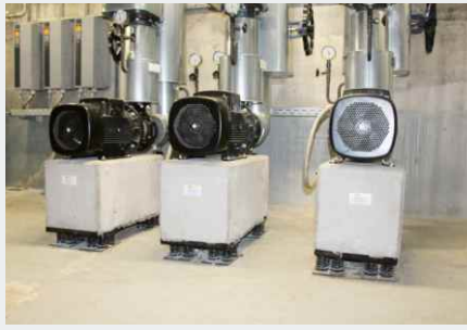
Bearing of pumps with additional mass
