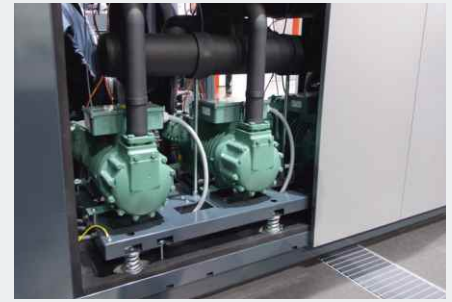
Industrial heat pump
