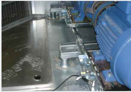
Bearing of belt-driven fans
