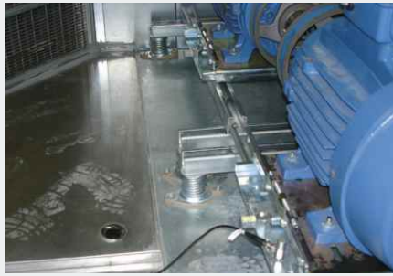
Bearing of belt-driven fans
