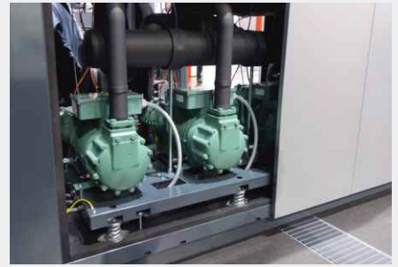
Industrial heat pump
