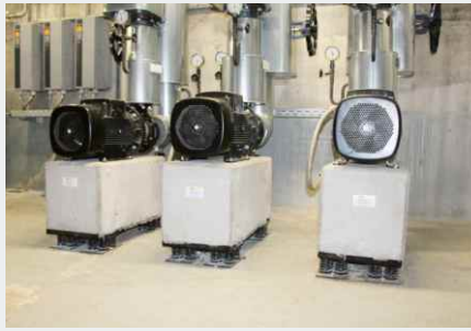
Bearing of pumps with additional mass
