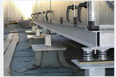
Roof-mounted AC system
