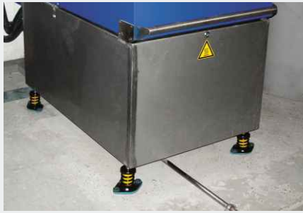
Small combined heat and power plant
