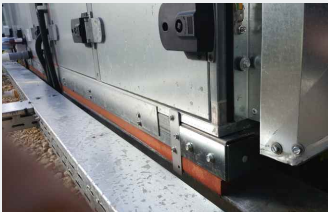
Strip bearing for air conditioning (AC) unit
