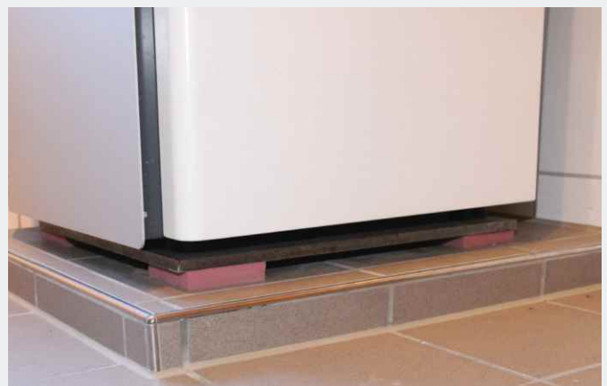
Decoupling of the internal unit of a heat pump
