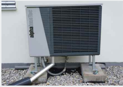
External unit heat pump
