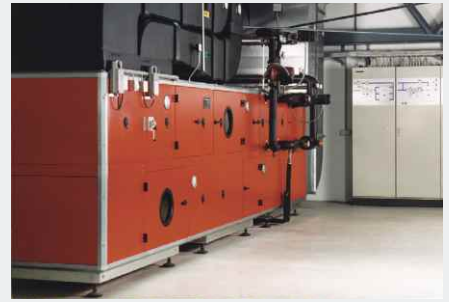
AC system installed in cellar
