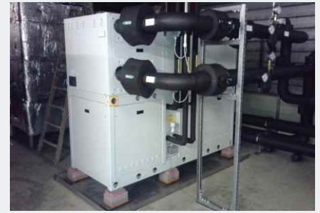
Chiller indoor unit
